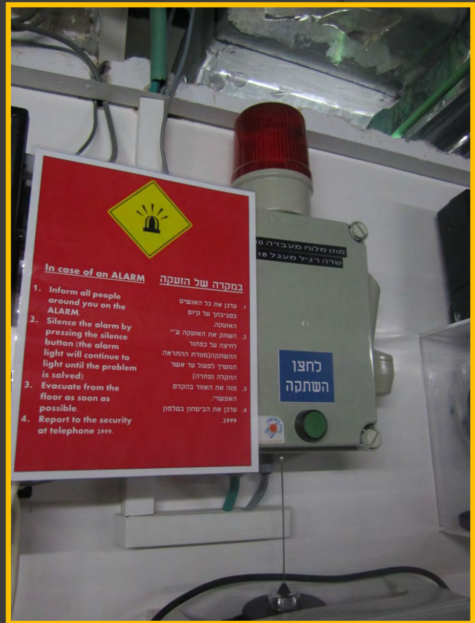
Alarm light and siren In the corridor
