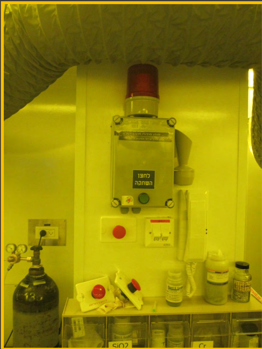
Alarm light and siren In the clean room
